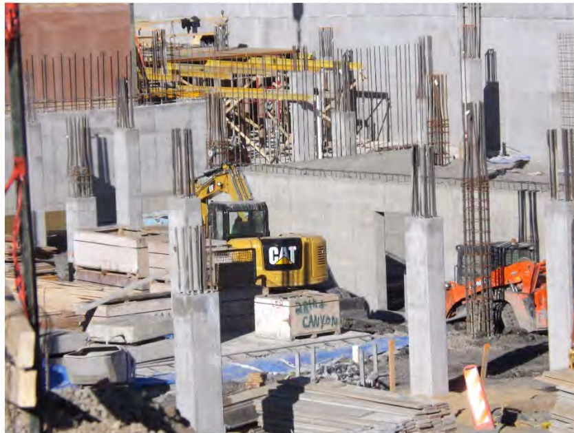
Figure 6 Concrete everywhere Hotels at 28 th and Canyon show need for extra concrete support pillars
