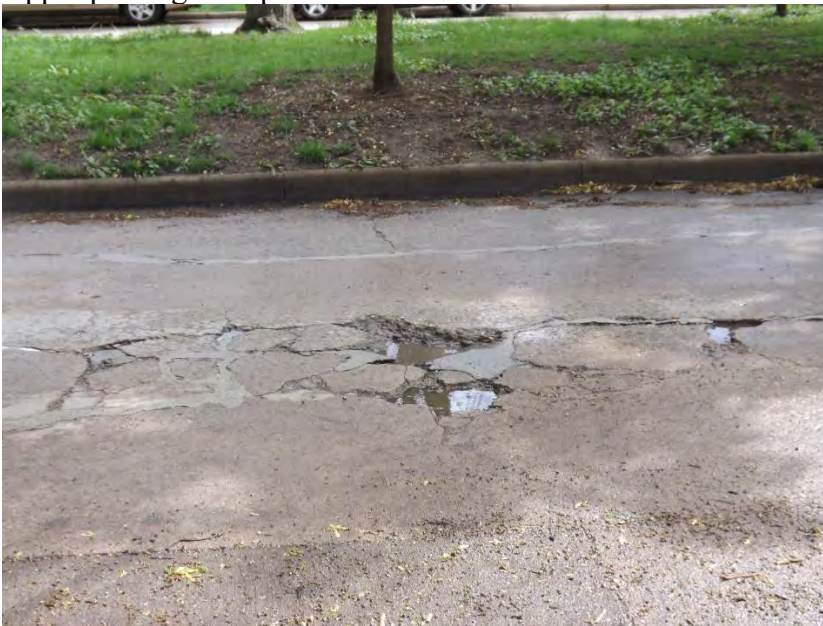
Mapleton Ave is breaking up 6th and Mapleton 4/27/2017
