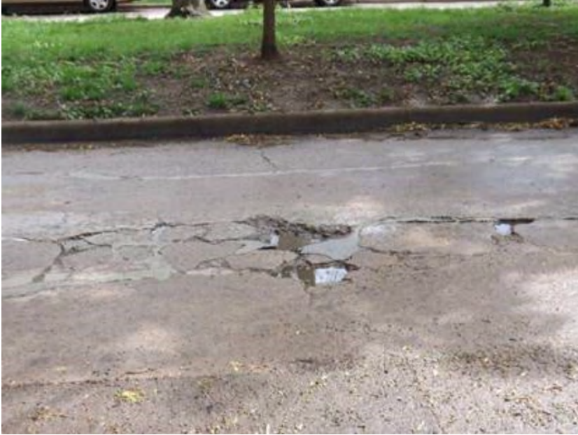
Mapleton Ave is breaking up 6th and Mapleton 4/27/2017
