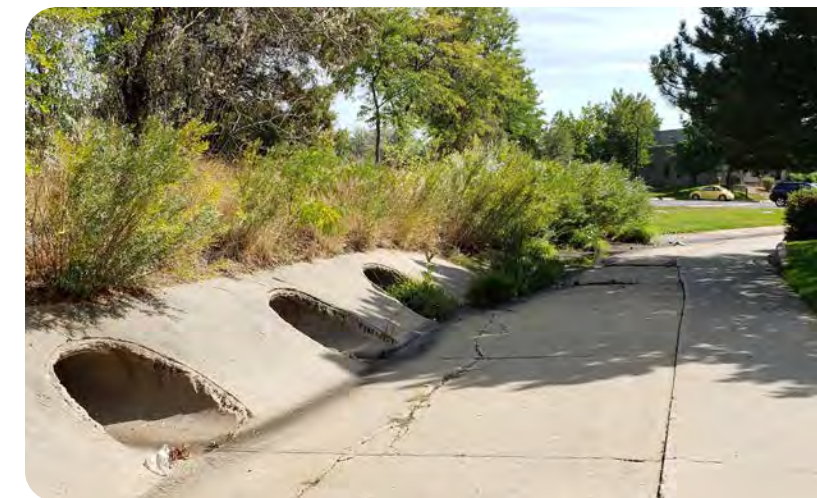
Flatirons Park Stormwater Drainage
