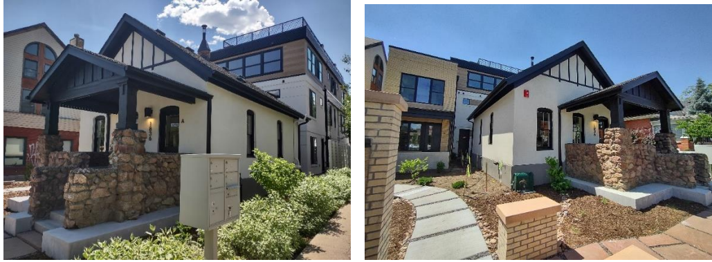
Figure 1. Left: northwest corner of 1836 Pearl St., showing the relocation of the building, new construction at the rear and rehabilitation of the historic building including the stone front porch, windows, door, and stucco. Right: The northeast corner of the rehabilitated building with the new construction beyond.
